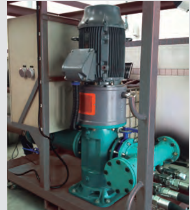
Asphalt Refinery 530 gpm / 120 m 3 /h 150 psi / 10 bar Heating system
